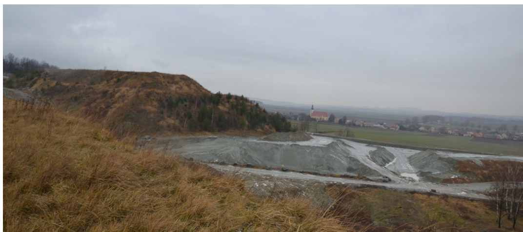
Figure A2. Mining waste treatment facility of the Gabbro Mine “Braszowice” – on the left: completed, on the right: under construction (photo U. Kaźmierczak, 2017).
