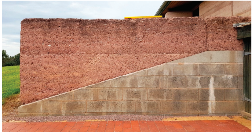
Figure 8. Wall 1 seen from the west. Note the accumulation of eroded debris at the base of the wall.
