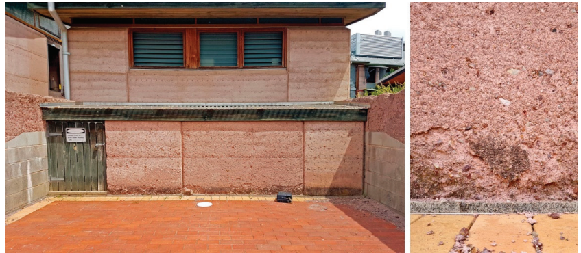
Figure 20. Paved space between wing walls 3 (left) and 4 (right) of Building 762. Note the decay at the base of the wall of the composting chamber.
