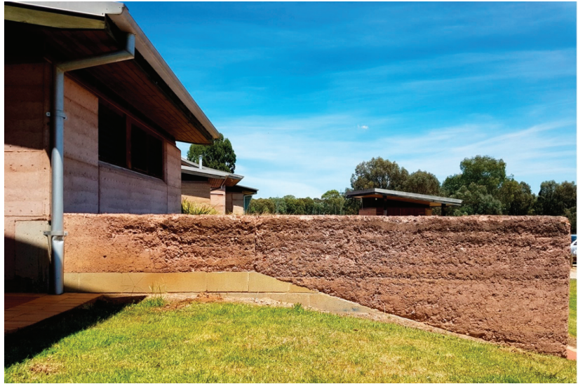
Figure 10. Wing wall 3 seen from the east. Note the linear decay at left, indicating different layers of compaction.
