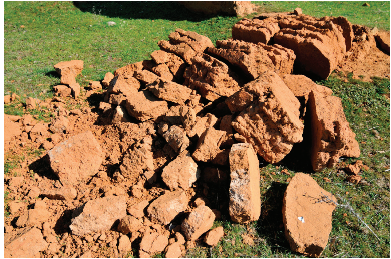
Figure 2. The collapsed southeastern block as seen from the southeast on 30 September 2015. Note the clean breaks and lack of bonding between the compaction layers. Reprinted from Ref. [9].
