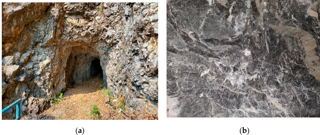
Figure 2. Photos of the surrounding rocks in the entrance and trunk sections: (a) surrounding rocks at the portal and (b) surrounding rocks in the trunk section.
