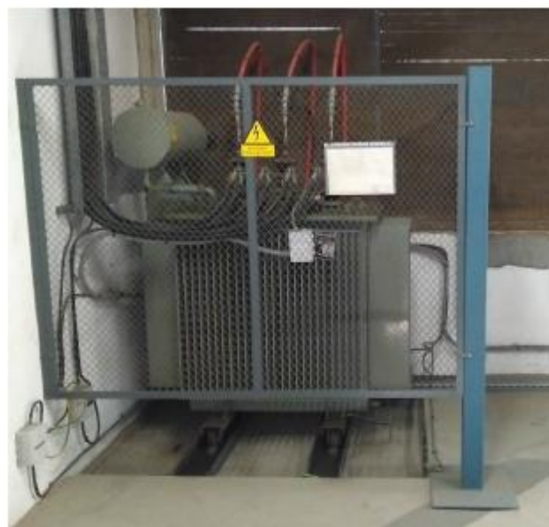
Figure 5. Example of a distribution transformer studied to test the developed model.
