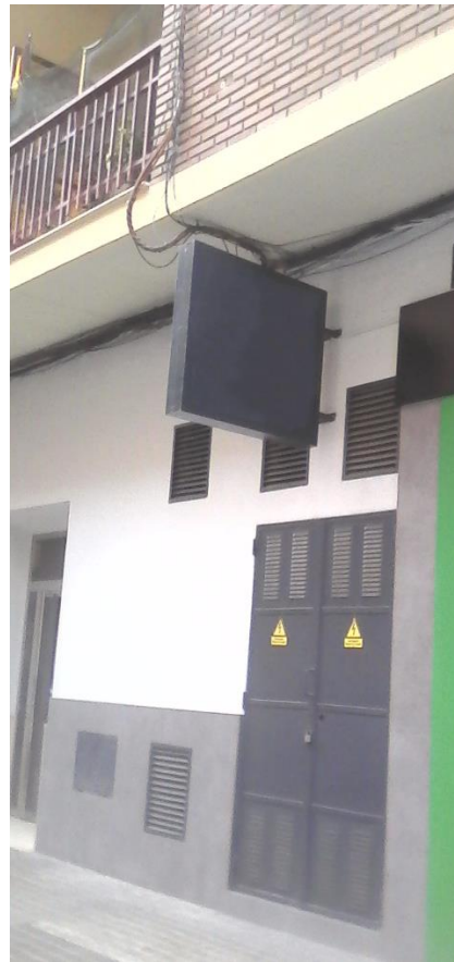
Figure 9. Location of the studied distribution transformer substation (DTS) in a building.
