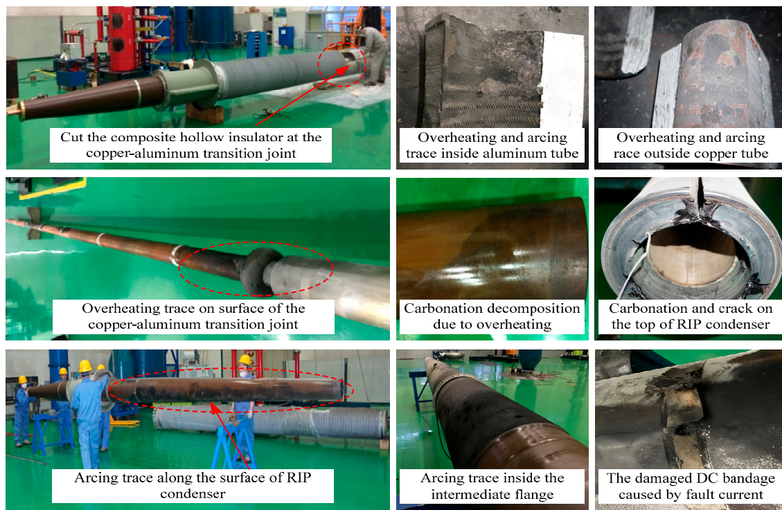
Figure 4. Arcing and overheating trace detected on the RIP condenser and conductive tube.
