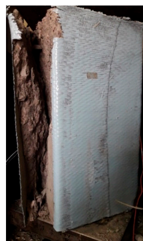
(iv) Pre-damaged and Hybrid strengthened
