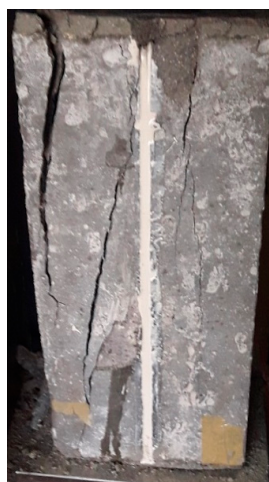
(iii) Pre-damaged and NSM strengthened
