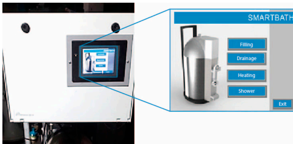
Figure 4. Electronic system and interface (controller).
