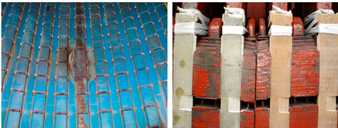
Figure 4. Damaged internal windings of the generator.
