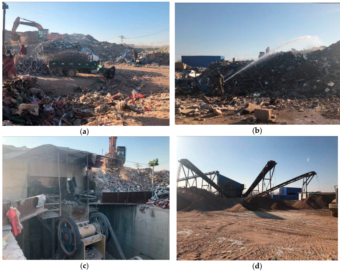
Figure 1. Subgrade filler preparation process: (a) eliminating clutter; (b) sprinkling; (c) crushing; (d) screening.
