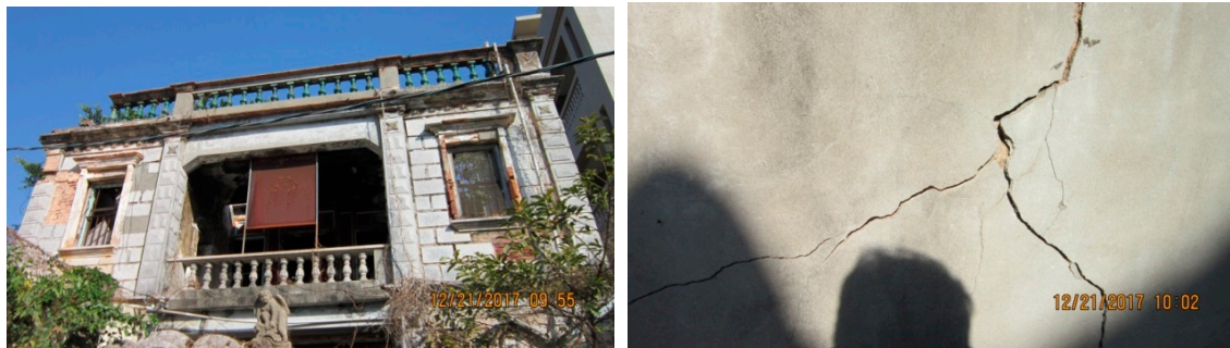
Figure 2. Historic western architectural house (left) and its damaged concrete wall (right).
