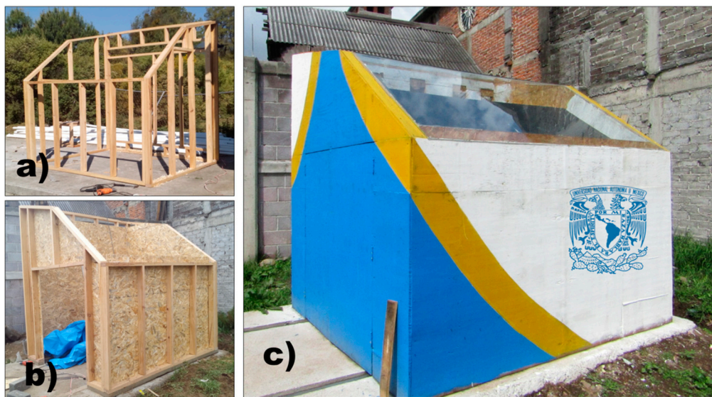
Figure 11. Construction of the solar dryer: (a) structure, (b) cover walls, (c) Finished construction.
