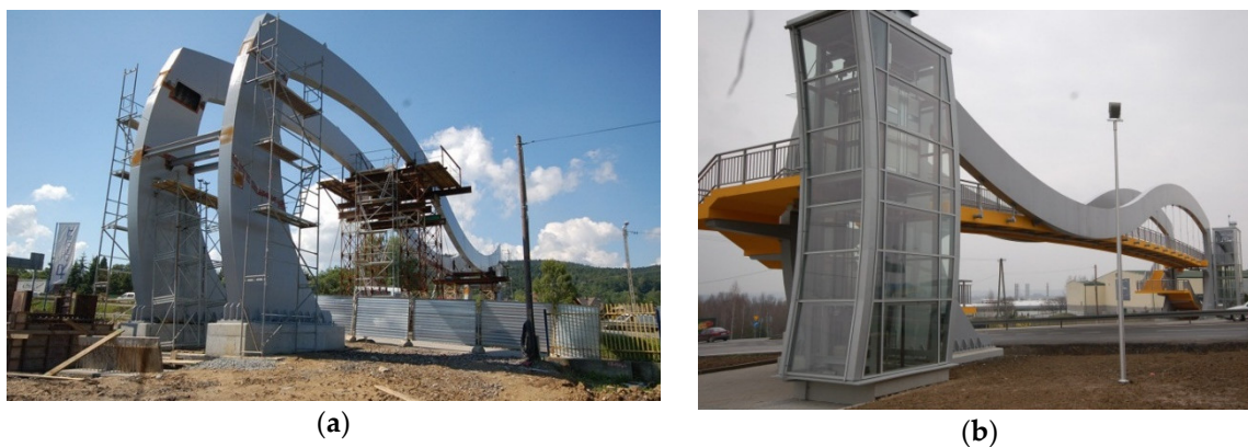
Figure 3. The footbridge structure: (a) steel frame during the montage, (b) the footbridge after assembly [18].
