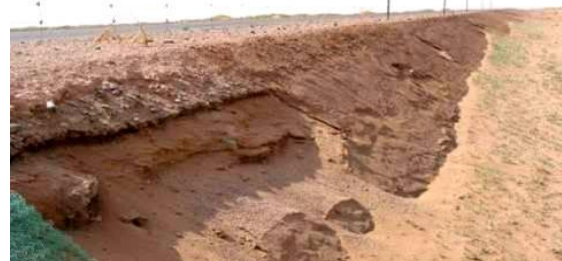
(b) Severe wind erosion of grassland soil due to traffic
