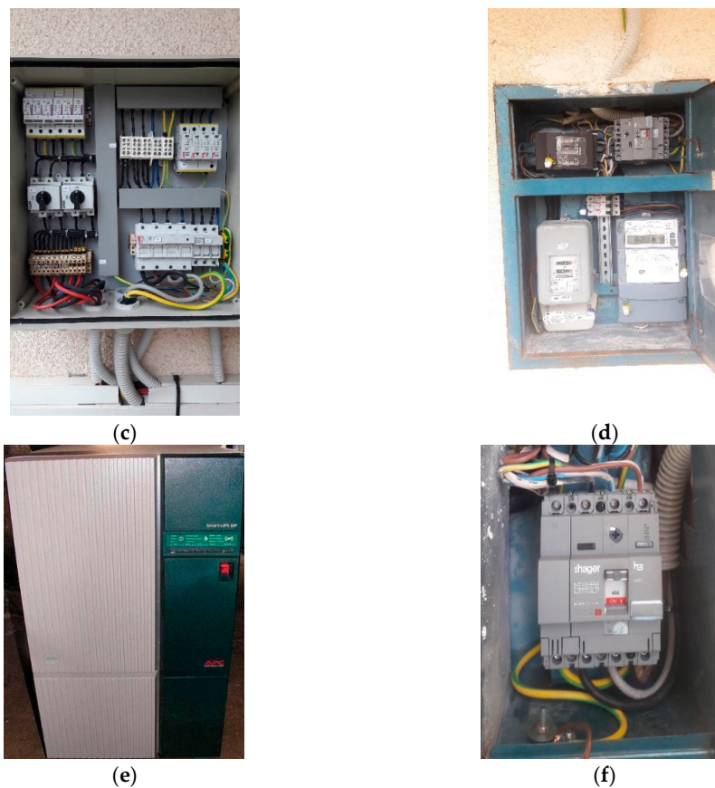
Figure 19. (a) PV plant on house, (b) electrical cabinet and inverter, (c) electrical cabinet for AC installation, (d) smart meter with line breaker, (e) smart UPS, and (f) line breaker.
