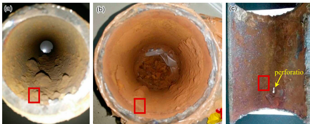
Figure 2. Corrosion morphology on the internal walls of steel pipe sections: (a) 2" pipe, (b) 4" pipe and (c) 6" pipe.
