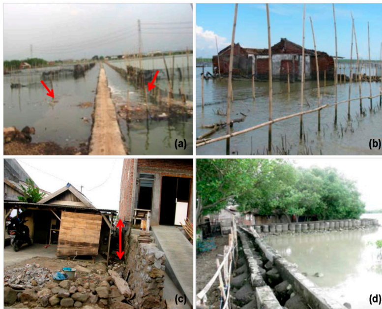
Figure 2. Some impacts of coastal erosion, inundation and subsidence in the study area: (a) Eroded land alongside the elevated road (red arrows show the initial width of the road); (b) inundated houses; (c) a house with an elevated floor; and (d) embankment and mangrove for coastal protection.
