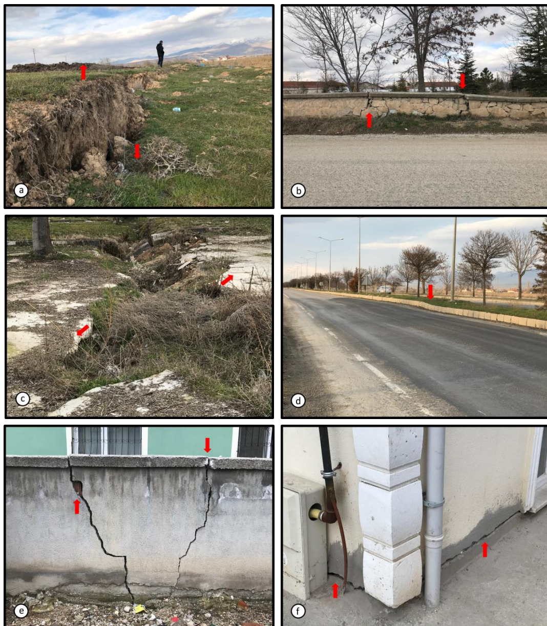
Figure 1. Ground deformations observed in Bolvadin and their effects on land, roads and structures.
