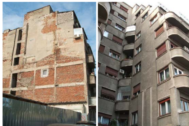
Figure 10. High-rise apartment building, with RC columns and beams, infilled with masonry, erected before 1940. Left side: a building without visible strengthening or renovation. Right side: with local repair, that is, limited and inadequate jacketing of columns, after 4 March 1977 earthquake.
