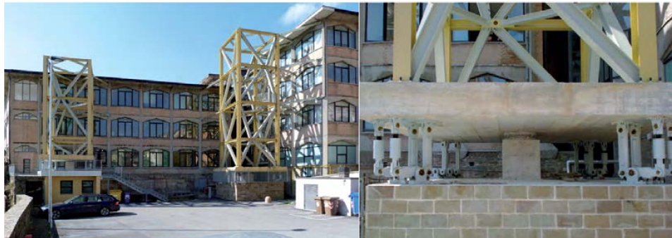
Figure 8. Retrofit intervention by means of dissipative towers and viscous dampers in Camerino (Macerata) [80].
