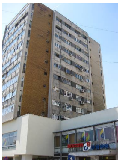
Figure 11. High-rise apartment building erected in the 1970s, having commercial spaces at ground-floor, with visible damages from 4 March 1977 earthquake, before renovation.
