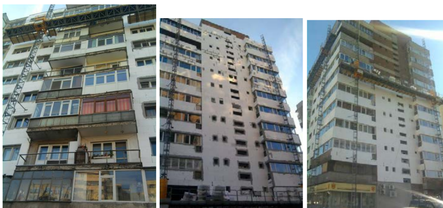
Figure 22. Large high-rise apartment building in Bucharest, erected in the 1970s, during energy renovation.
