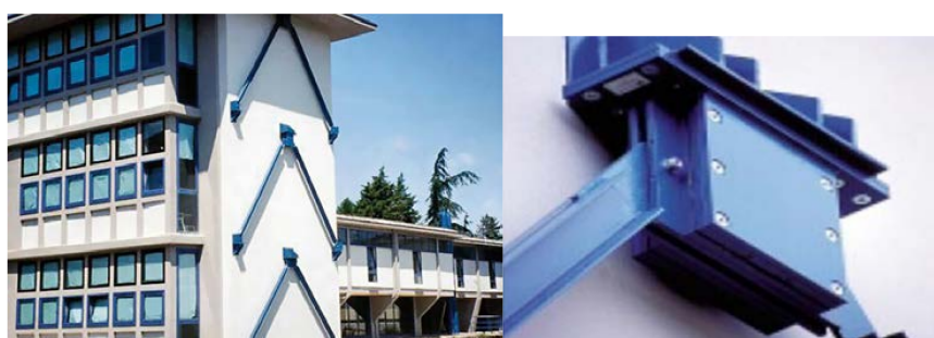
Figure 7. Retrofit intervention by means of viscoelastic dampers in the school Gentile-Fermi in Fabriano (Ancona) [71].
