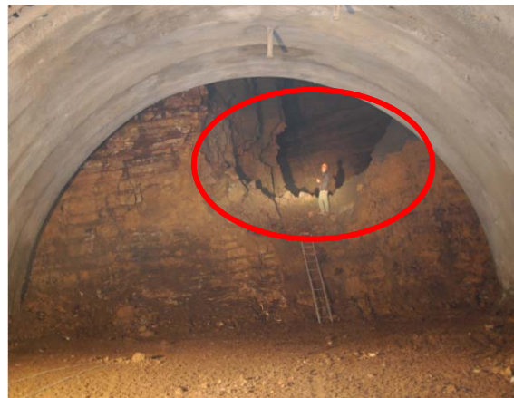
Figure 5. Revealed karst cave on the tunnel face.
